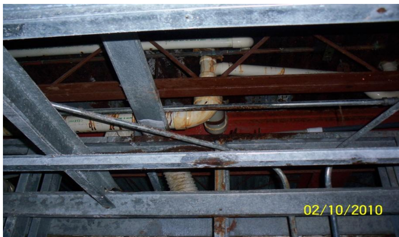
226 PIPE BURST CAUSING FLOODING IN LOWER UNIT
